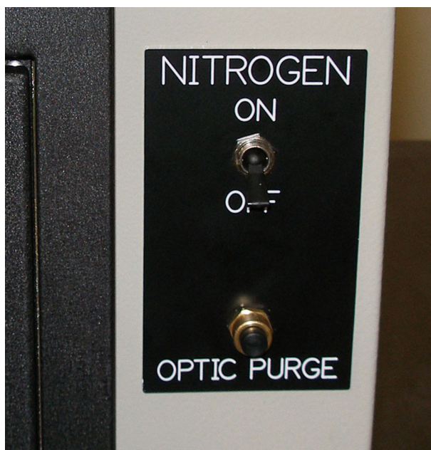
Figure 2-23, Sulfur Optic Control Panel
